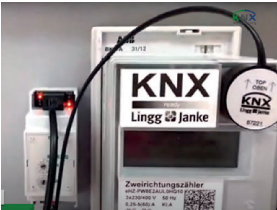
The optical head reads the data from the meter and transmits it to the KNX bus, as indicated by the red illuminated LED at the top left.
